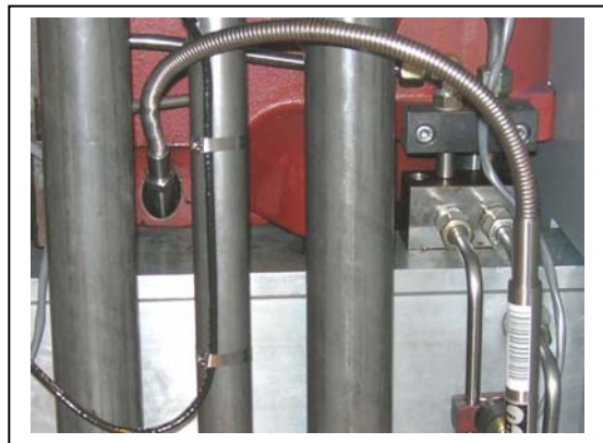
Fig.4: Installation place of HTT-Sensor
