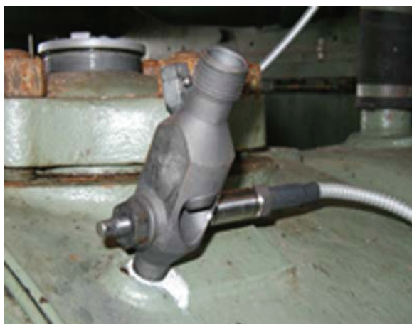
IPT-01XHT sensor installed on Kiene valve
