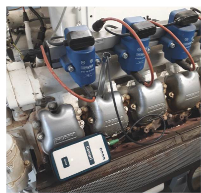
Compri installed on a power plant MAN E2842 Le312 4-stroke gas engine
