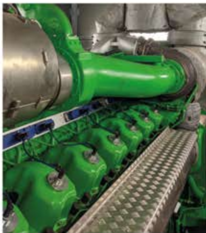
Currently the ISP-01 spark plugs are successfully tested on a Jenbacher engine type 6
